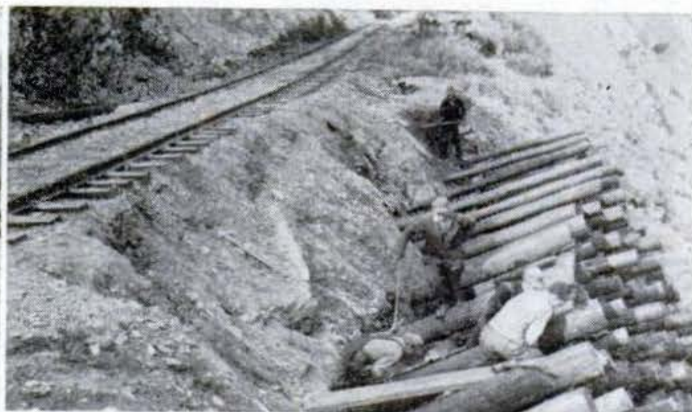
SIXTY-FOOT PILINGS , pounded into the road-bed at an angle (above), help to support track on thawing mountain as soil shifts. This section of track has to be rebuilt each year.
